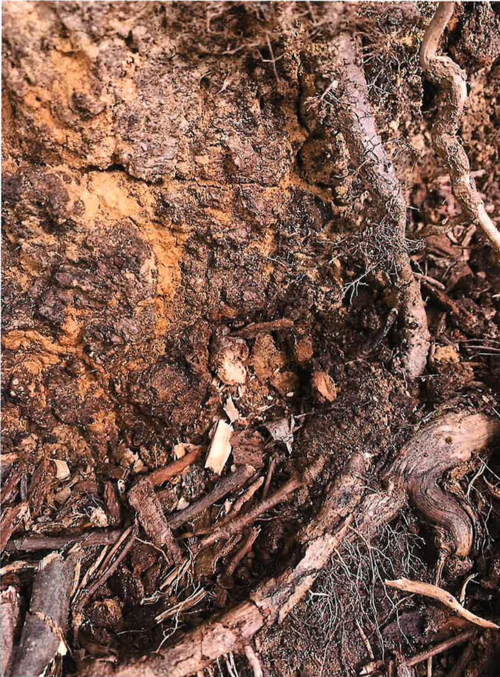
Image 16. Debris stuffed into a bore hole in Tree T46 in an effort to conceal it from detection. Photograph taken by Mark Tan on March 1, 2022.
